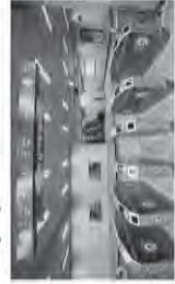
Line 9 transfer gate
